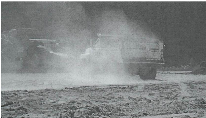
Unmitigated dust emanating from ongoing heavy equipment operation at Woodlands (Sep. 2013).
