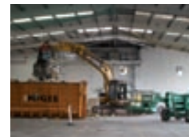
Portal frame building due to be reclaimed by Portal Power on a London regeneration project
