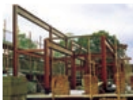
Reclaimed steel re-fabricated and reused at no extra cost saving 178 tonnes embodied CO 2
