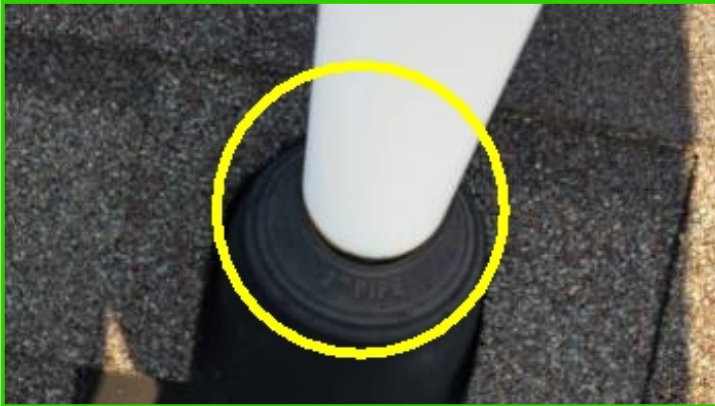
Replace seal or cover with sleeve. Obvious gap on rubber.
