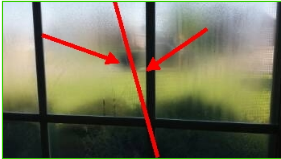
Window is cracked and needs to be replaced. Estimated cost is $200
