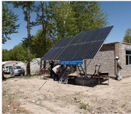
15KW Photovoltaic water pumping for Agricultural Irrigation Wulan, Qinghai,
