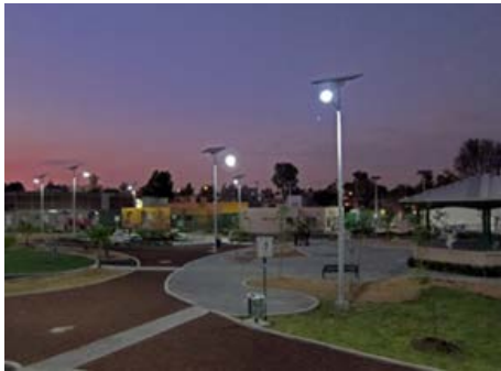
Type of PV Street Light : Pole Top Type Site location: Surabaya, Indonesia.
