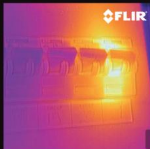
Overheated connection (with MSX)
