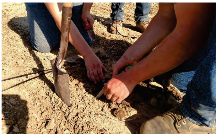
Installation of the soil moisture and temperature sensor in furrow in 2017.
