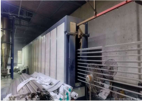
Heat chamber UNIT 1
