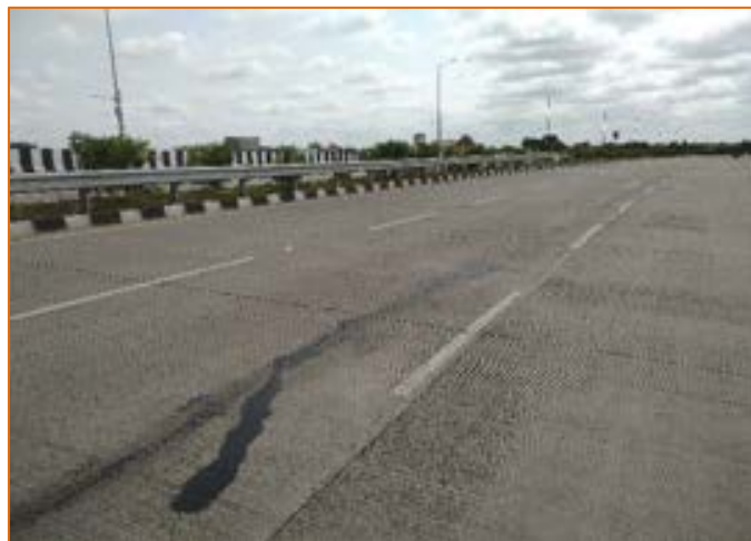
Pavement Condition at km. 287+700 (RHS)
