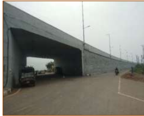
VUP at km. 432+050 (LHS) - (Miyani) under COS - RE Block Wall at A1 side
