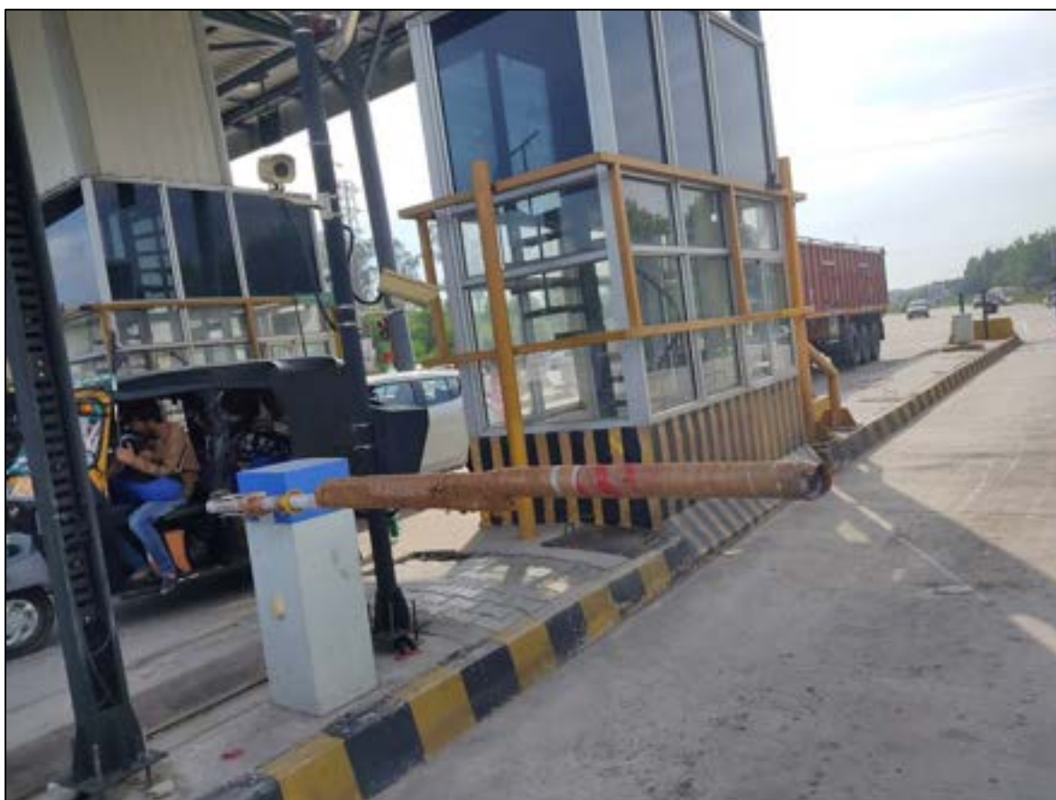
Figure 9-7 Automatic Lane Barrier
