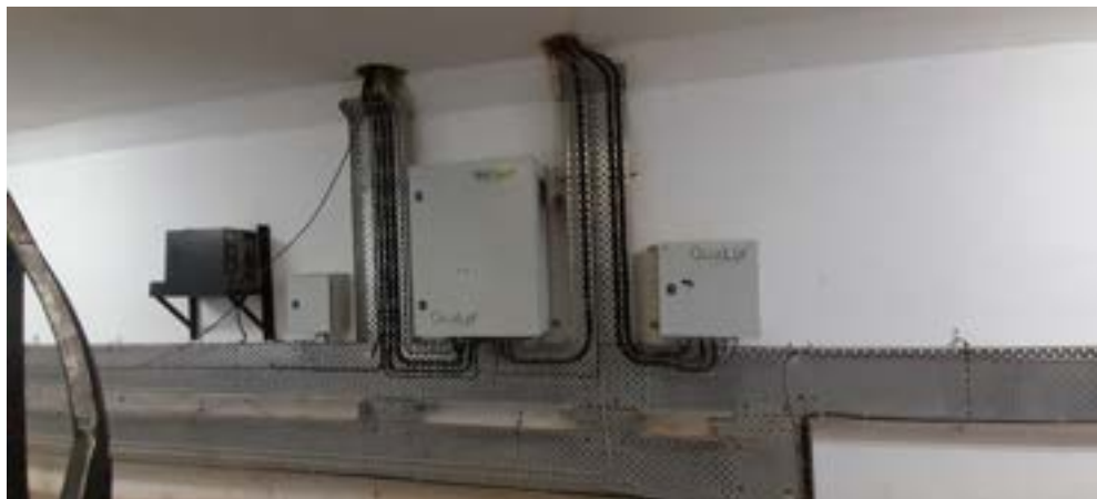
Figure 9-3 Lane Controller and AVC installed in enclosures at Toll Booth
