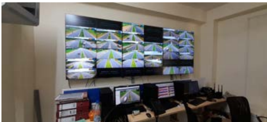
Figure 9-17 Video wall at ATMS Control room
