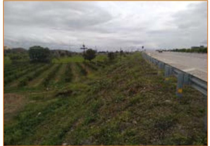
Crash Barrier at High Embankment Location
