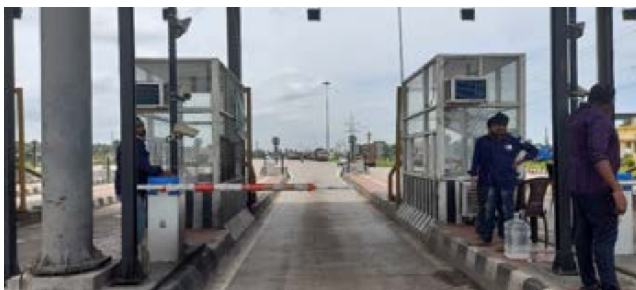
Figure 9-6 Automatic Lane Barrier
