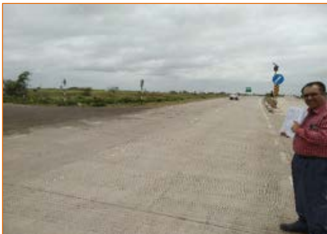
Pavement Condition at km. 306+500 (LHS)
