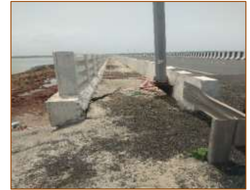
Major Bridge - km. 433+295 (RHS) Footpath settled
