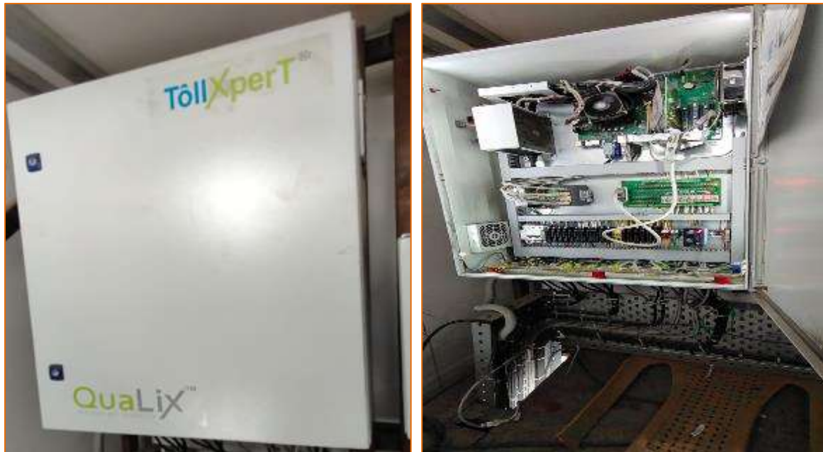
Figure 9-3 Toll Lane Controller TLC
