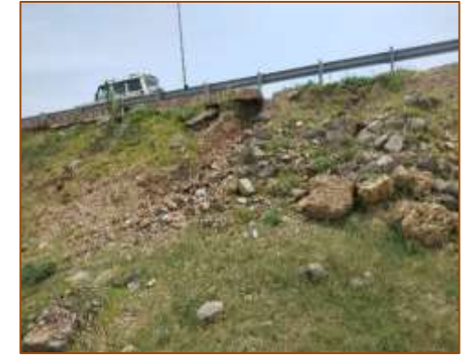
Rain cuts developed at A2 side at MJB at km. 415+929 (RHS)
