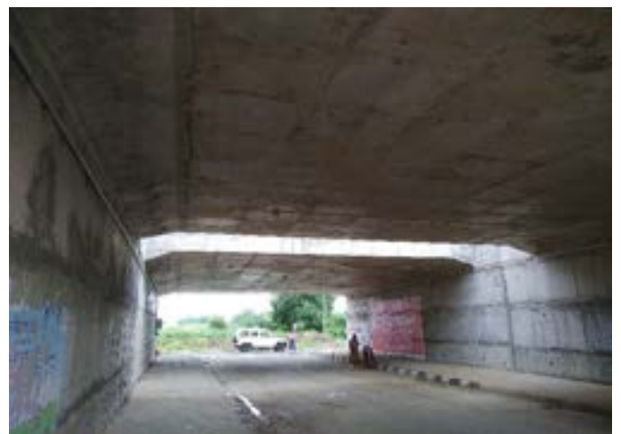
Lighting arrangement made under structures
