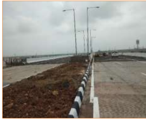
Wearing Coat of VUP at km. 12+420 (BHS)
