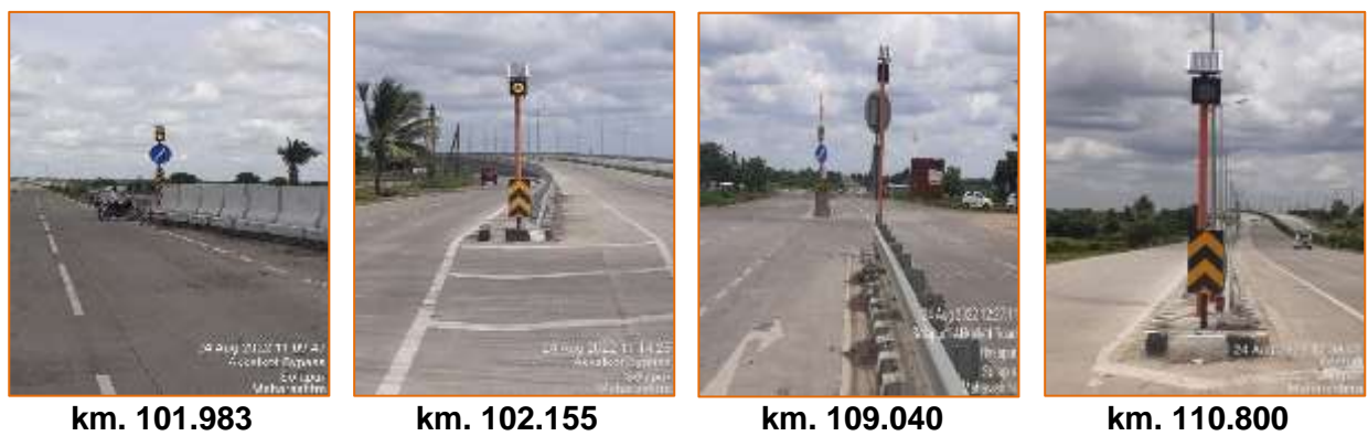
Figure 3-11 Photographs of Highway/Solar Lighting
