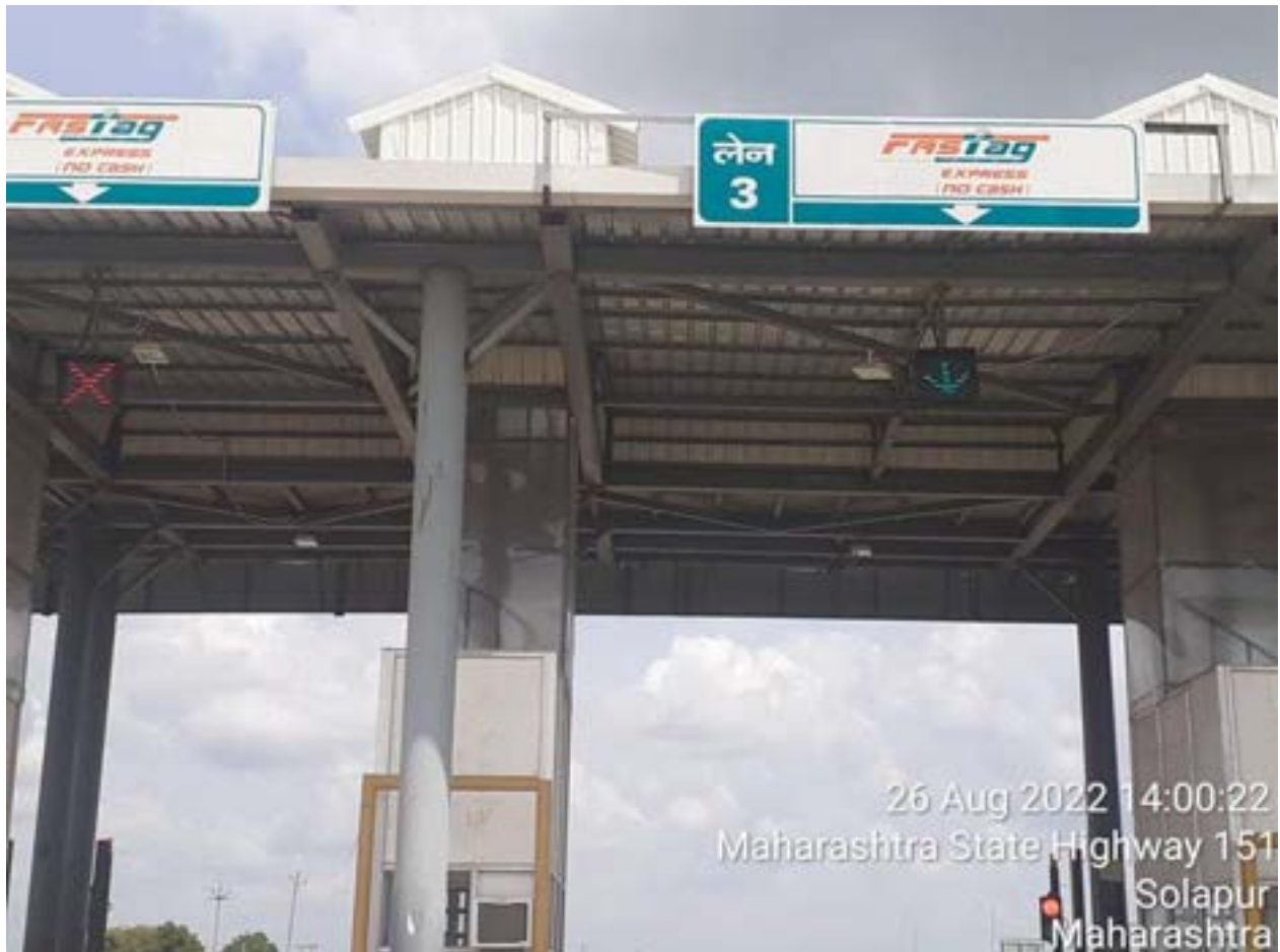
Figure 9-5 OHLS indicating green arrows for operational lanes
