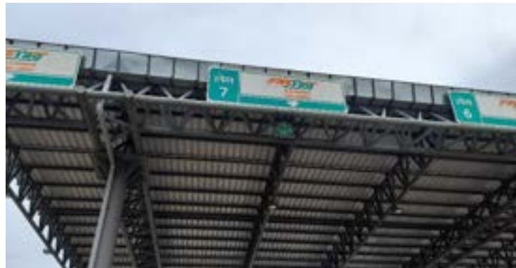
Figure 9-9 Over Head Lane Signal (OHLS)
