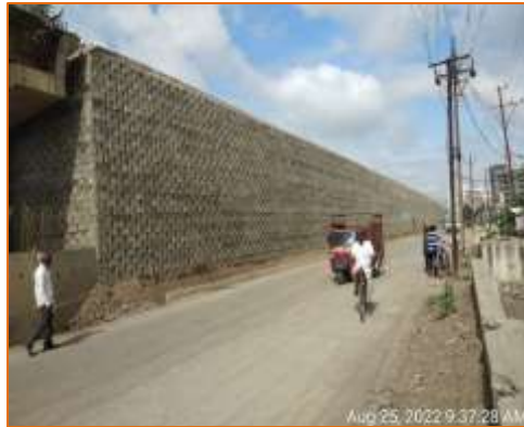
Friction slab & crash barrier of Flyover pending at km. 136.857 @ A2 side (RHS)
