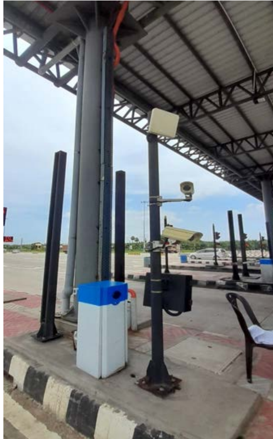
Figure 9-2 RFID ETC Transceiver installed on pole
