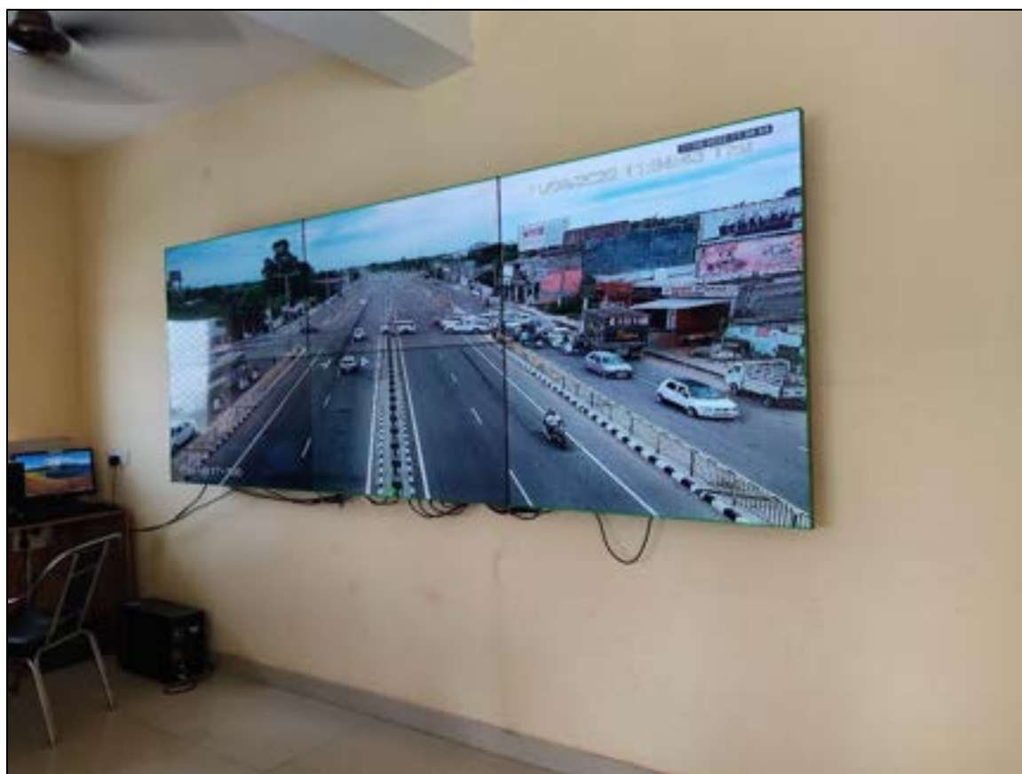
Figure 9-18 Video wall at HTMS Control room
