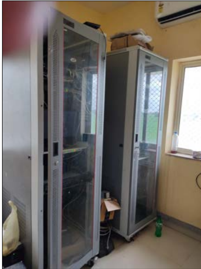
Figure 9-13 Control Room Equipment - Server & Switch rack
