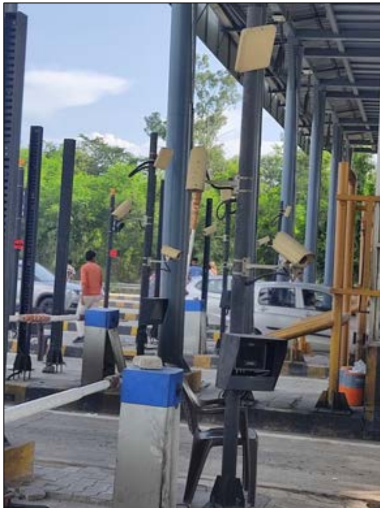
Figure 9-3 RFID ETC Transceiver installed on pole
