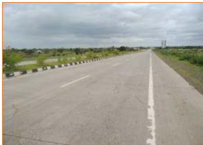
Pavement Condition at km. 319+100 (RHS)
