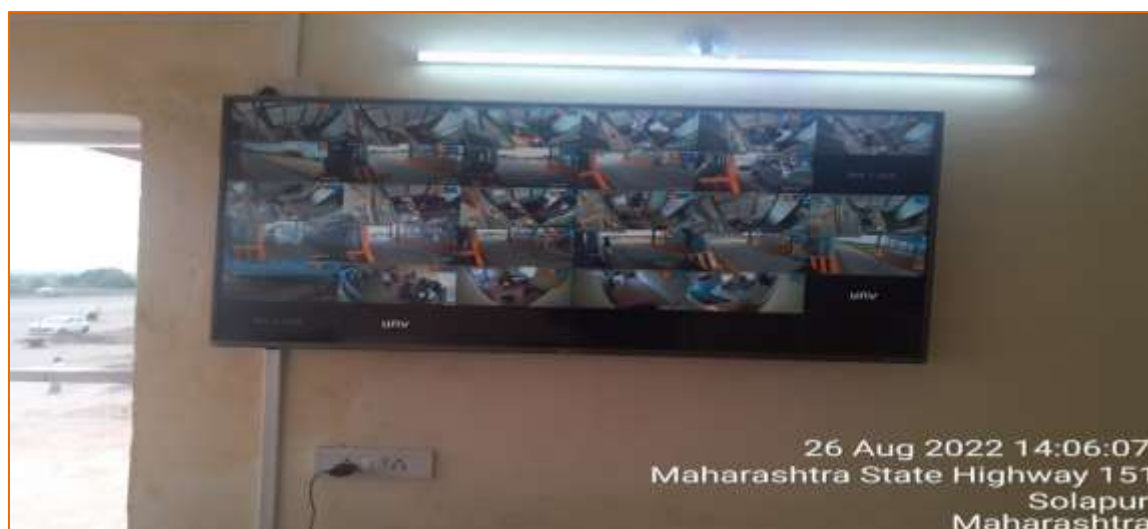
Figure 9-9 CCTV screen at the Toll Plaza Control Room
