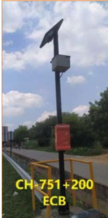
Figure 9-6 ECB at km. 751.200
