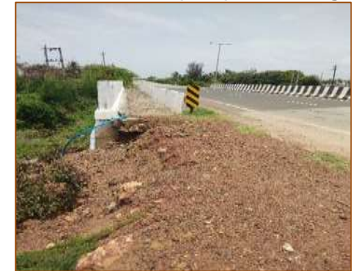
Side View of Minor Bridge at km. 440+350 (LHS) - Rain cut developed
