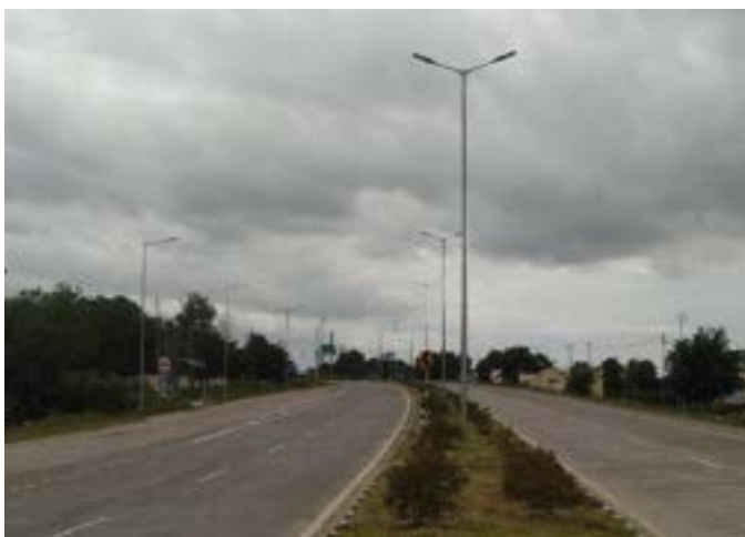
Highway Lighting at km. 313+700
