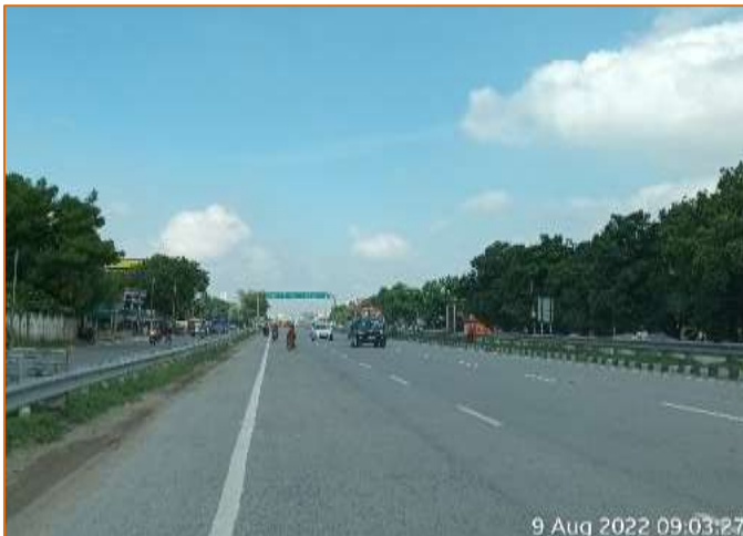
Pavement Condition at km. 785+200 (RHS)
