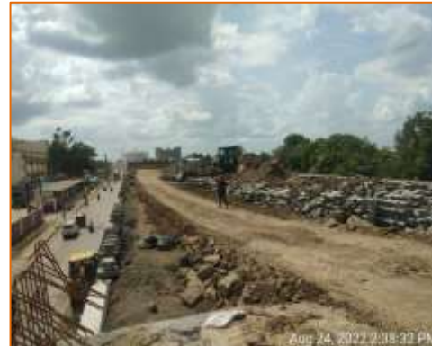
Filling work & RE Block erection work of Flyover is in progress at km. 136.857 @ Akkalkot side (LHS)
