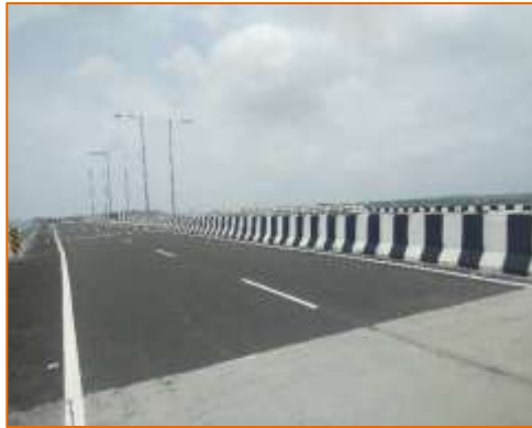
Wearing Coat of ROB at km. 0+527 (RHS)
