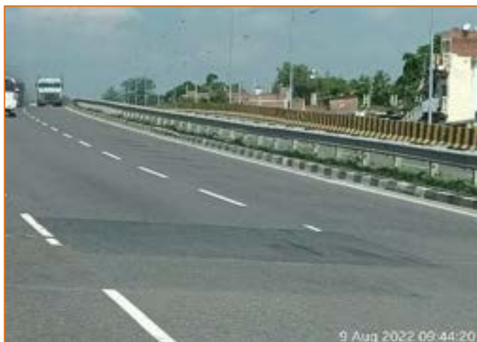
Pavement Condition at km. 765+100 (RHS)
