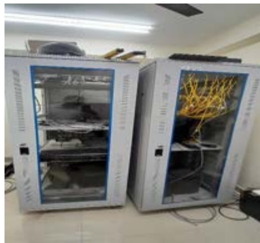
Figure 9-12 Control Room Equipment - Server & Switch rack
