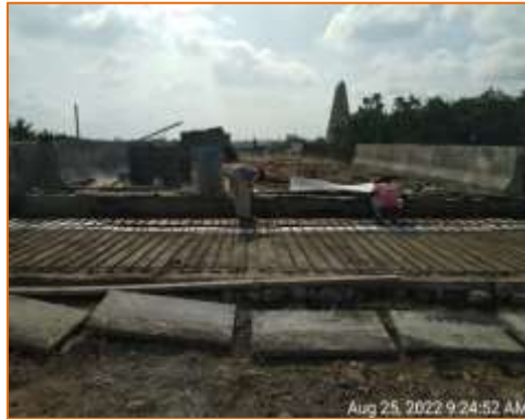
Approach slab work @ A2 side of Flyover is in progress at km. 136.857 (LHS)
