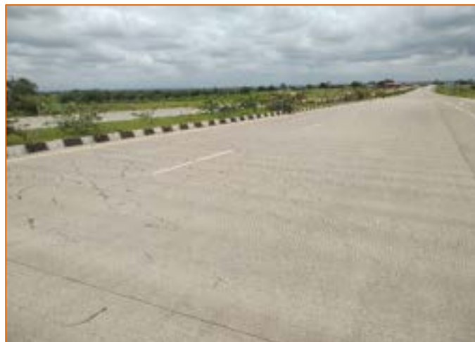
Pavement Condition at km. 304+600 (LHS)
