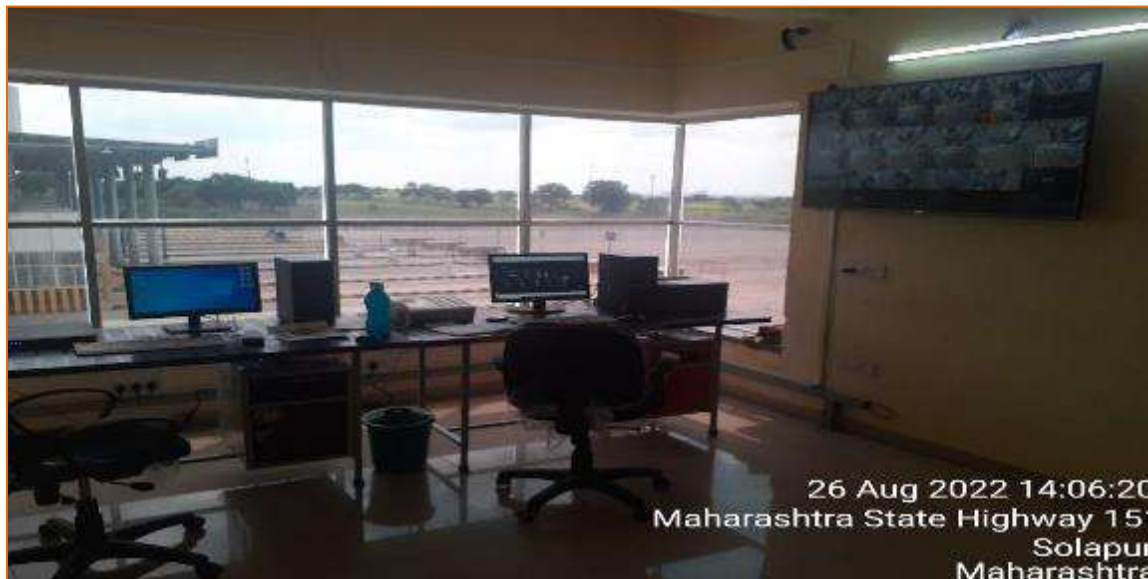
Figure 9-10 Incident Management Workstation at Control room
