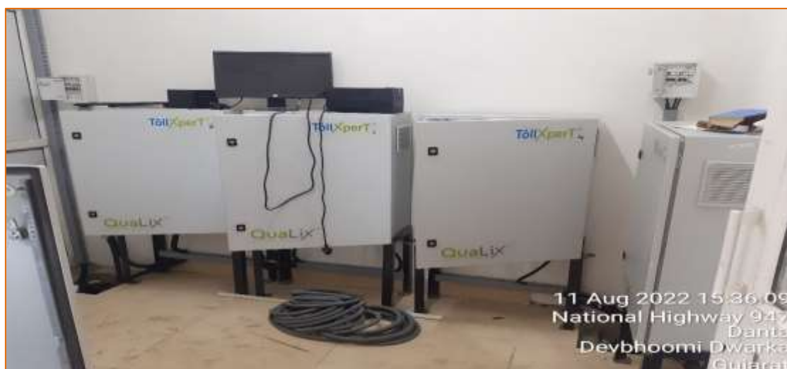
Figure 8-3 Lane Controllers for normal ETC lanes
