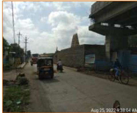
RE Block wall & FSCB of Flyover pending at km. 136.857 @ A1 side (RHS)
