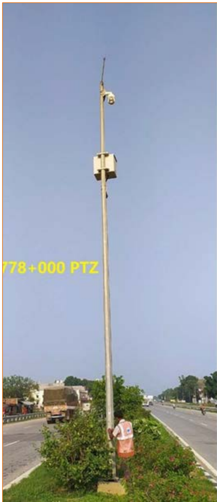
Figure 9-9 PTZ camera at km. 778.000
