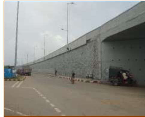
VUP at km. 432+050 (LHS) - (Miyani) under COS - RE Block Wall at A2 side
