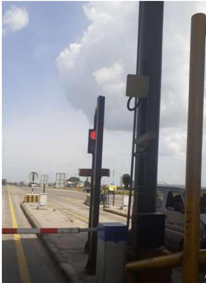
Figure 9-2 RFID ETC Reader mounted on Pole
