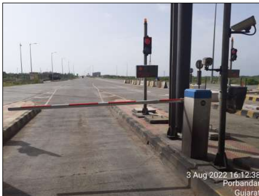
Figure 9-6 Automatic Lane Barrier
