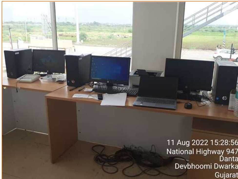
Figure 8-10 Workstations at Control room
