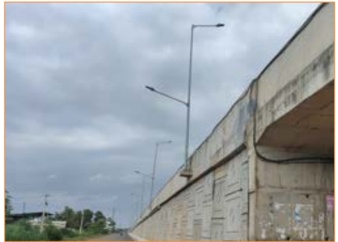
Highway Lighting at km. 44+135
