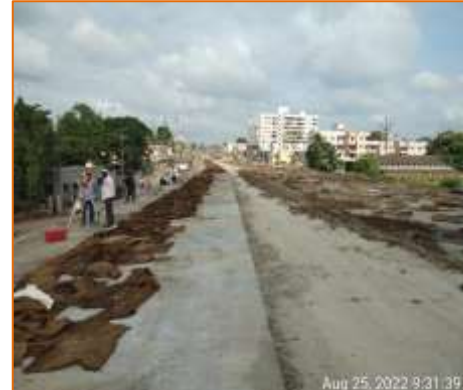
DLC & PQC of Flyover is in progress at km. 136.857 @ Solapur side (BHS)
