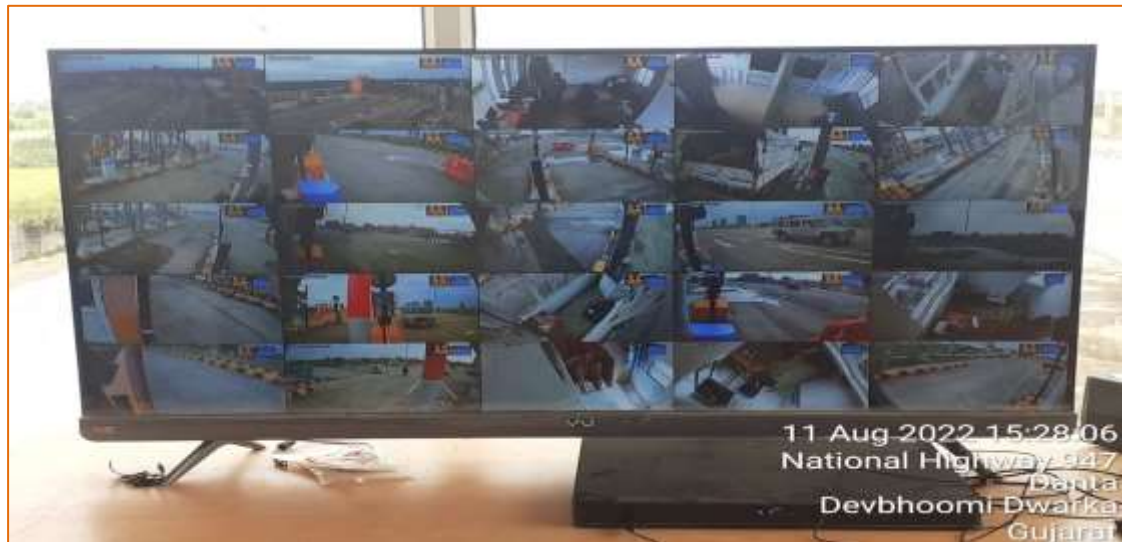
Figure 8-9 CCTV screen at the Toll Plaza Control Room
