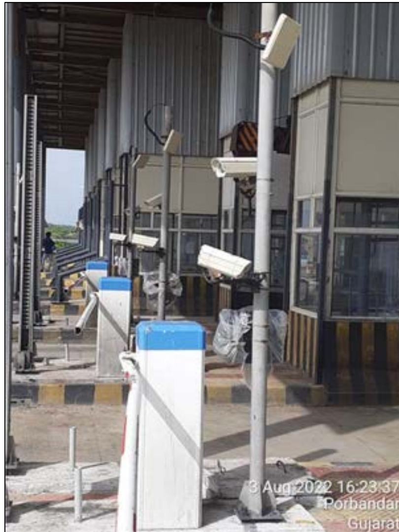
Figure 9-3 RFID ETC Reader mounted on Pole
