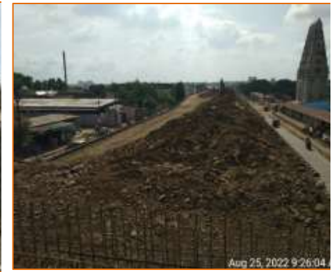
Filling work of Flyover is in progress at km.136.857 @ Akkalkot side (BHS)
