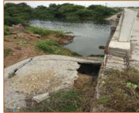
Damaged CC Pitching of MNB at km. 456+533 (BHS) on Both end
