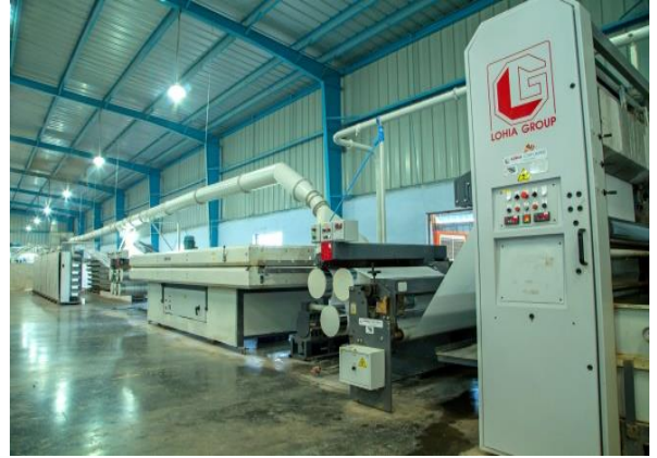
TAPE PLANT - II
