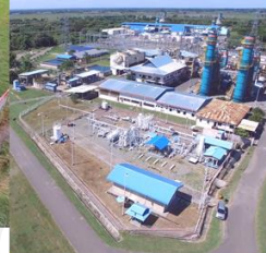
Patila Metering Station (PMS)
