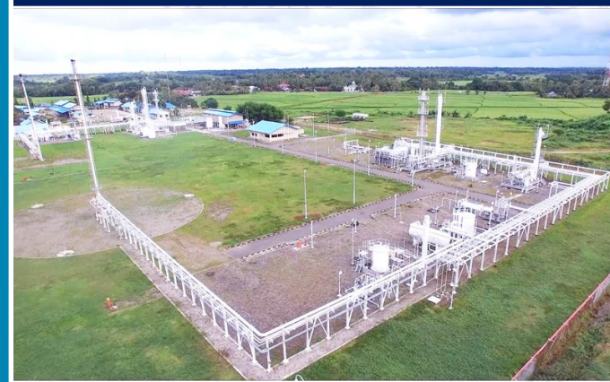
Central Processing Plant (Kampung Baru)
