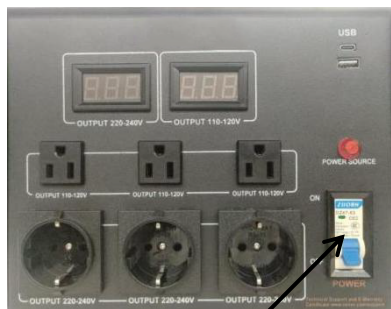
Power switch ( Air switch )
