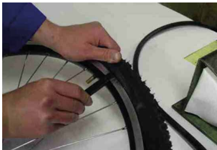
INCORRECT INSTALLATION / DISASSEMBLY
