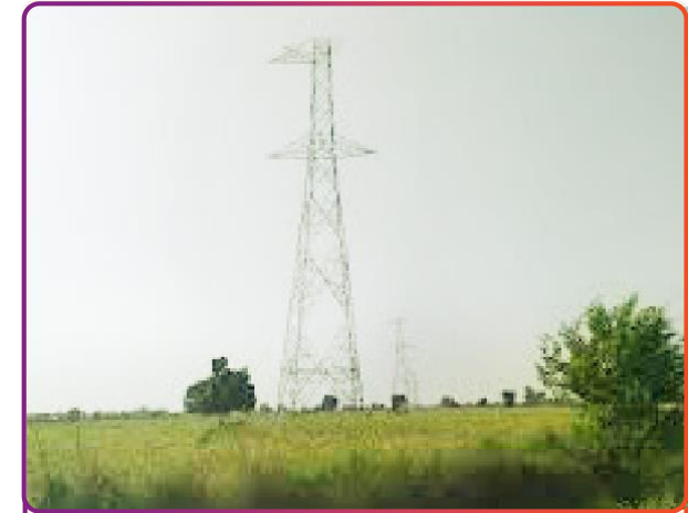
765kV Ghatampur TPS-Agra SC line
