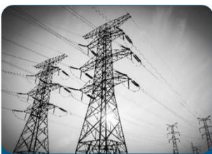
Longest Private HVDC Line in Asia
