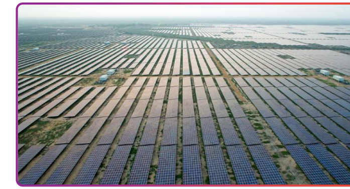
648 MW Ultra Mega Solar Power Plant (at Kamuthi, Tamil Nadu)
