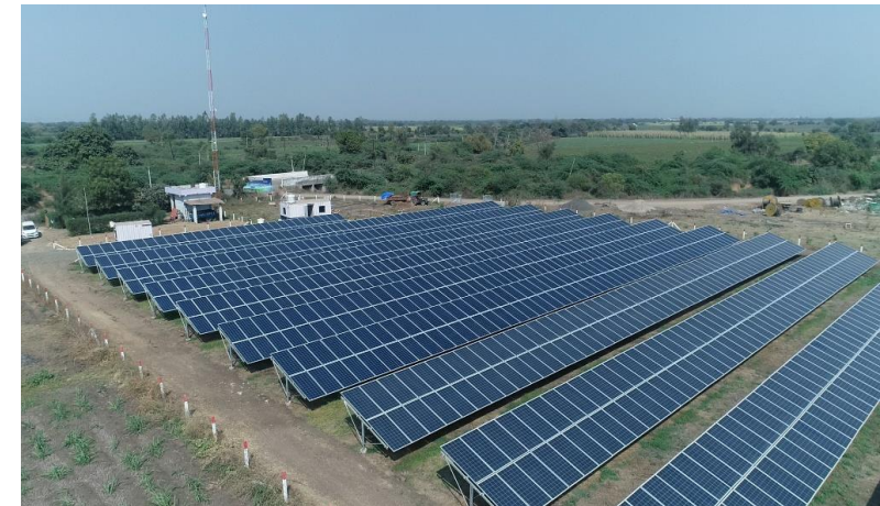
17.9 MW Solar plant installed at Bharuch
