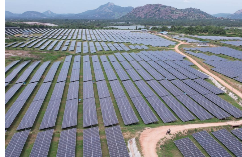
Solar panels (ground mounted)
