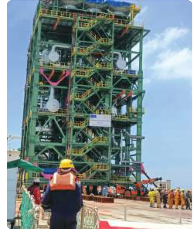
Linde New Gasification Plant Project at Kattuppalli Chennai by Asian Paints PPG (Contractor - L&amp;T Energy Hydrocarbon)
