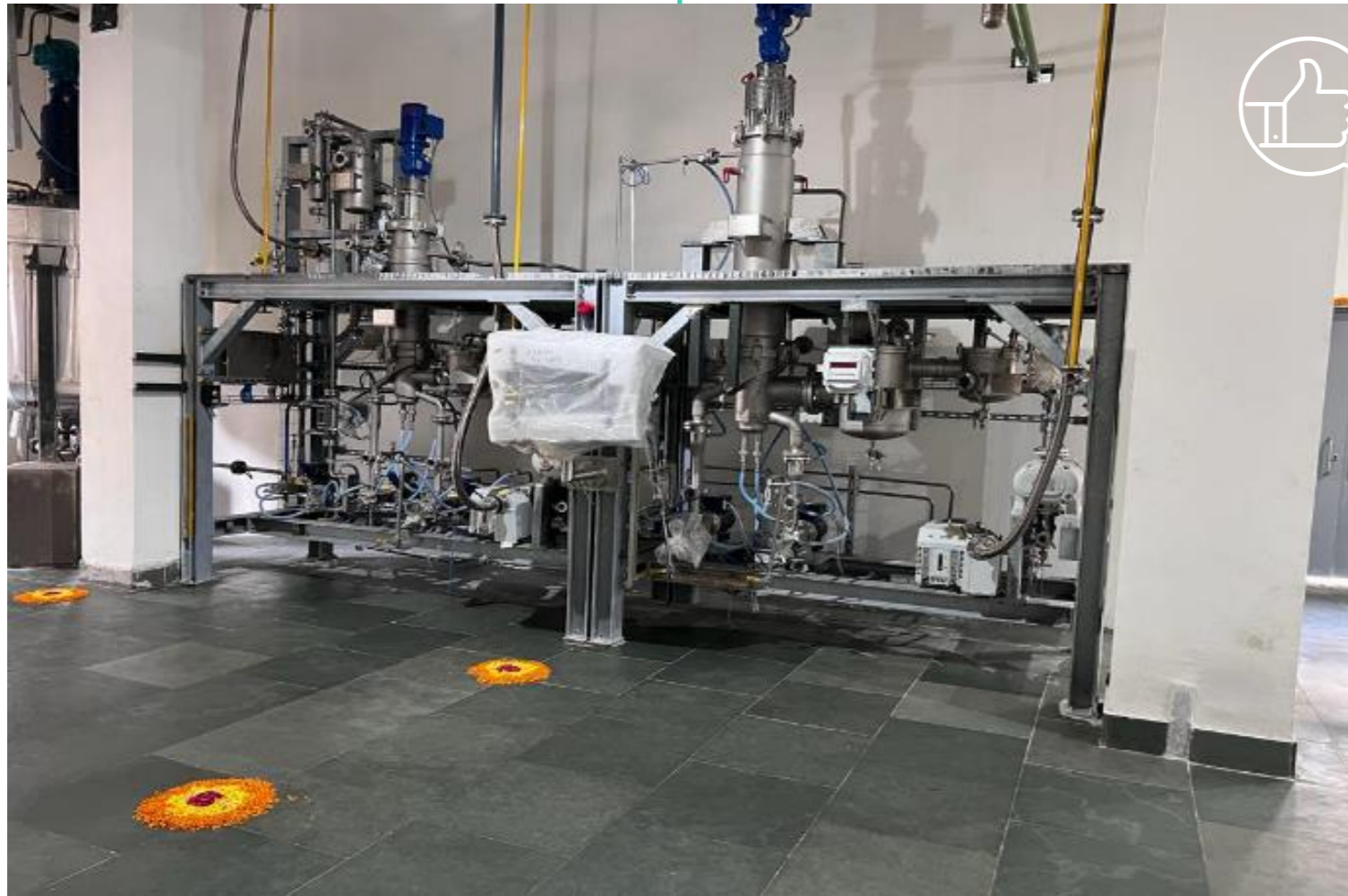
Commissioned operation in the SPDU plant of Polymers-Performance Materials Business
