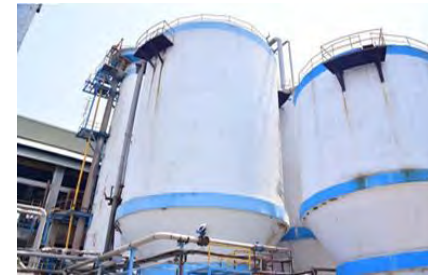
Fiber Line Pulp Mill
