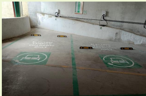
EV Charging station installed at Birla Centurion
