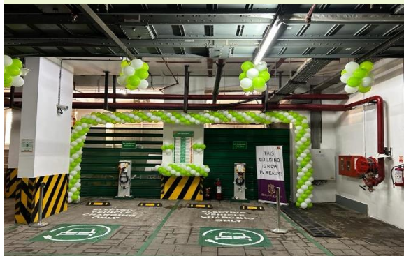
EV Charging station installed at Birla Aurora
