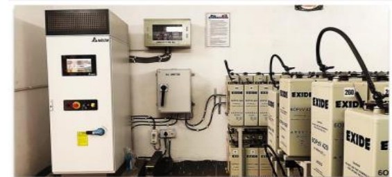
East Calcutta Substation (near Kakurgachi)
