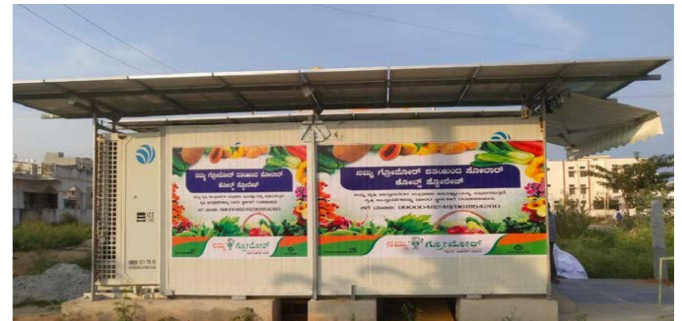
Ecofrost - Solar powered Cold Storage Room
