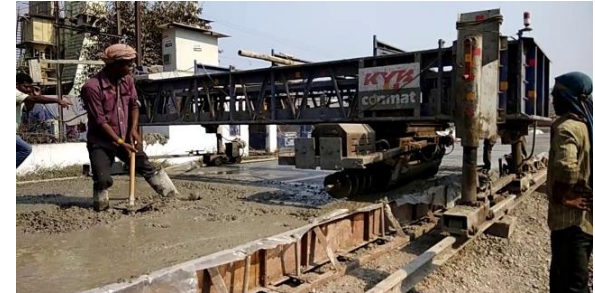
NHAI Project, Bihar & West Bengal Blended Cement usage in Pavement Quality Concrete
