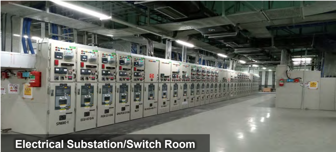
66/11 Kv GIS Substation
