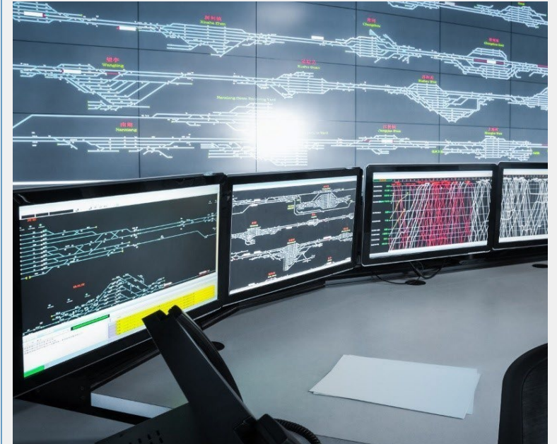
Implementing communication network including IP based Video surveillance system (VSS) for railways
