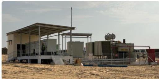
Invertor Control Room
