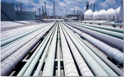
Anti Corrosive Material
