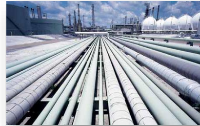
Anti Corrosive Material
