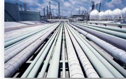
Anti Corrosive Material
