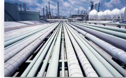
Anti Corrosive Material
