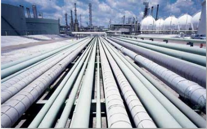
Anti Corrosive Material
