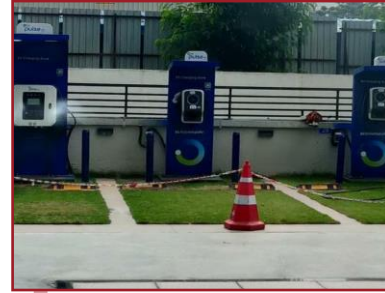
EV charging infra for employees
