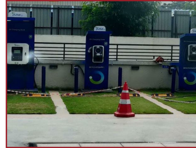
EV charging infra for employees
