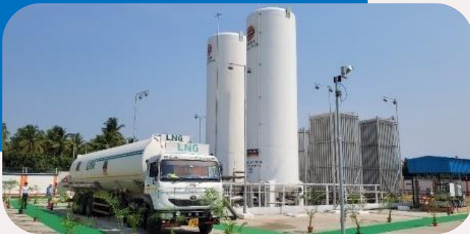
Order received from Adani Total Gas for 5 LNG Fueling station
