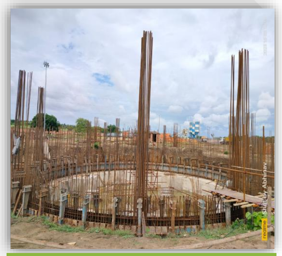
Cement Silo (MCS)
