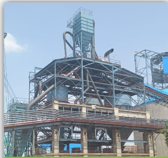
Cement Mill Hopper
