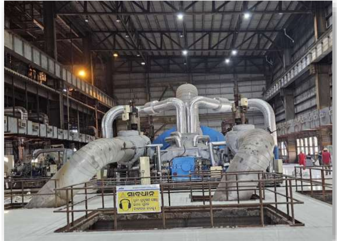
Unit 1 Turbine Generator set
