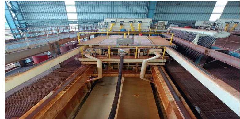
2 nd Filter Press at BPSL
