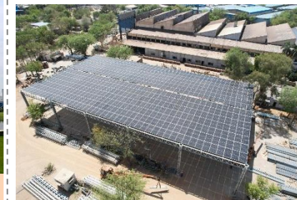
Solar rooftop plant
