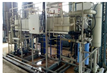
Acid Recovery Plant
