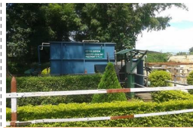
STP plant for waste water treatment
