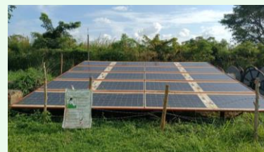
Solar panel installed at project sites
