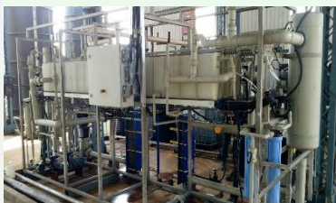
Acid Recovery Plant
