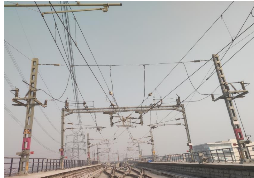
Overhead Electrification, Delhi Metro
