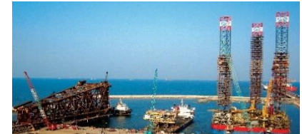
Fabrication Facility, Oman
