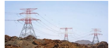
Transmission Lines, Fujirah, Dhaid
