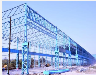
Viraj Steel Section Rolling Mill, Boisar
