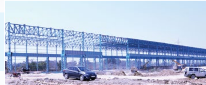
Viraj Steel Section Rolling Mill - Boisar
