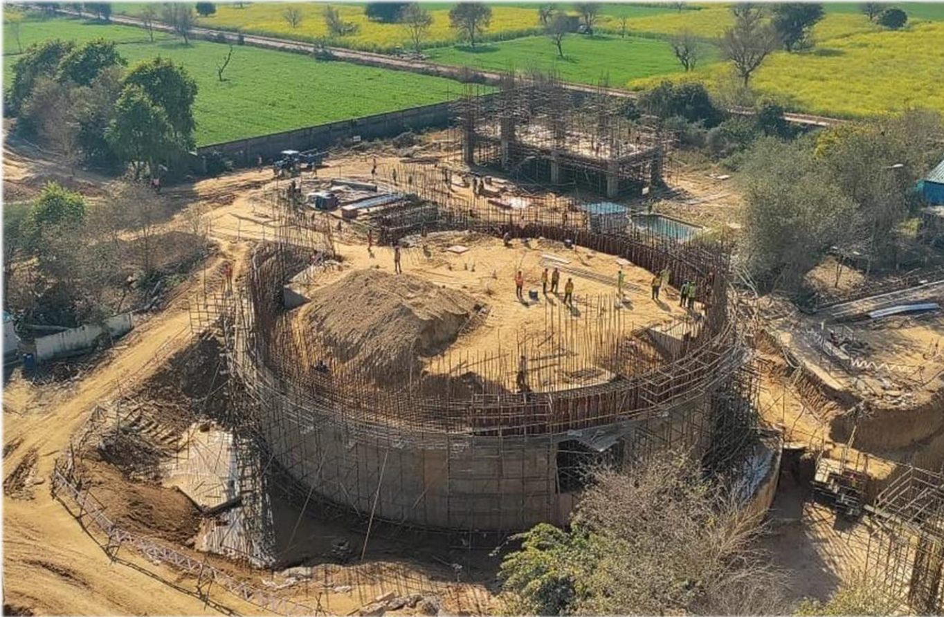
Clinker Silo, Bhiwani Cement Plant
