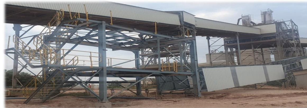
Additive conveyor for cement mill, Nimbol debottlenecking project
