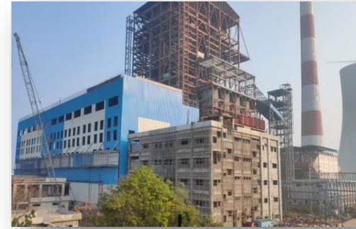
1x800 Mw TPSS, North Chennai, TNGEDCO
