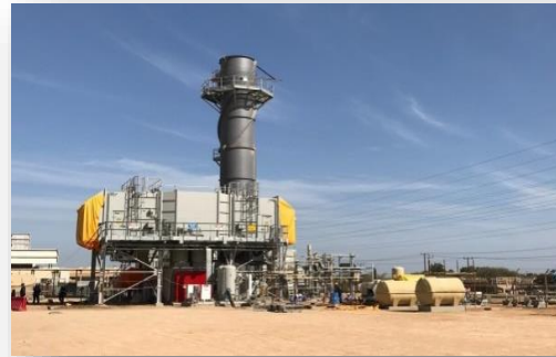
25 MW, Ray Project-RAY International LLC, Oman
