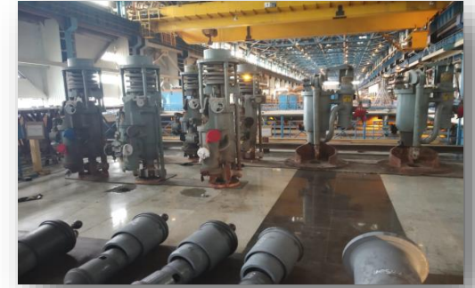
Control & Stop Valves Overhauling Sipat 660 MW
