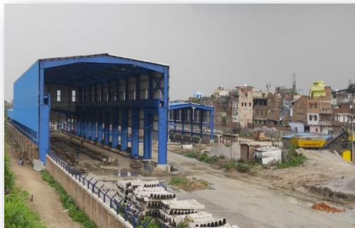
MEMU Shed at Kanpur-RVNL
