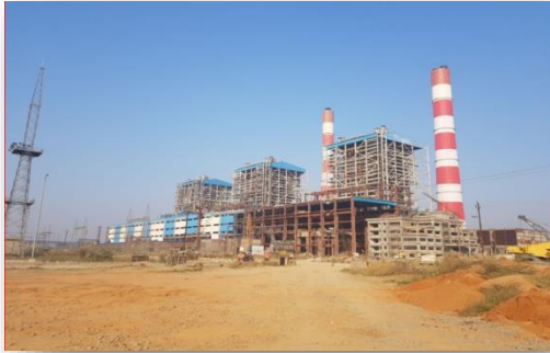
3x660 MW Nabinagar STPP, NPGCL
