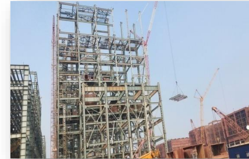
5x800 MW Yadadri TPP, TSGENCO
