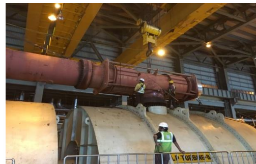
Turbine AOH, 600 MW, Udipi
