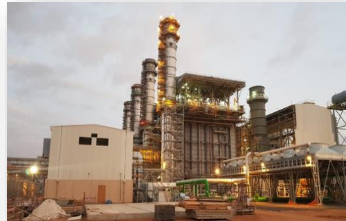
1,390 MW Waad Al Shamal ISCCPP, GE, KSA
