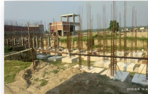
28 MLD STP at Karnal, TPL
