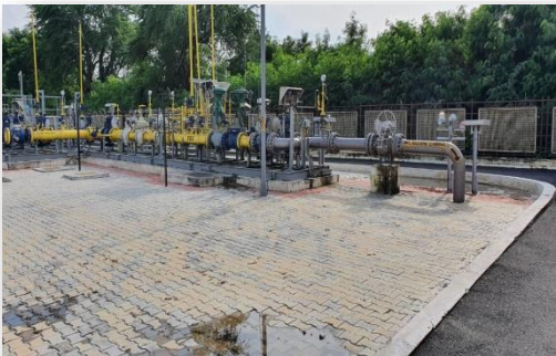
Station Piping at Ennore, IOCL
