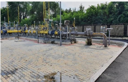
Station Piping at Ennore, IOCL
