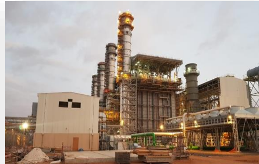
1,390 MW Waad Al Shamal ISCCPP, GE, KSA
