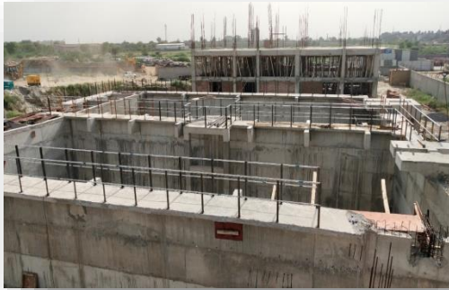
27.5 MLD STP, Networking at Palwal, MCPALWAL
