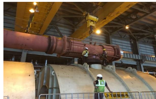
Turbine AOH, 600 MW, Udipi
