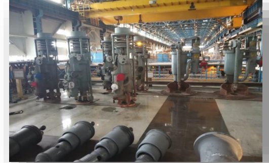
Control & Stop Valves Overhauling Sipat 660 MW
