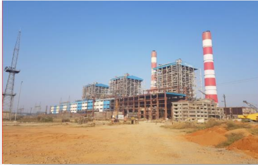
3x660 MW Nabinagar STPP, NPGCL
