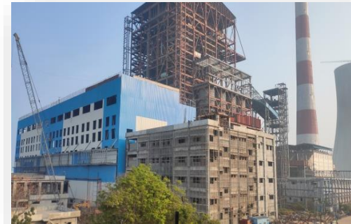
1x800 Mw TPSS, North Chennai, TNGEDCO
