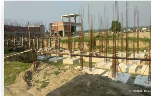
28 MLD STP at Karnal, TPL
