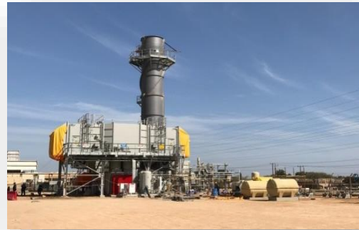
25 MW, Ray Project-RAY International LLC, Oman
