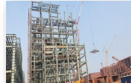
5x800 MW Yadadri TPP, TSGENCO
