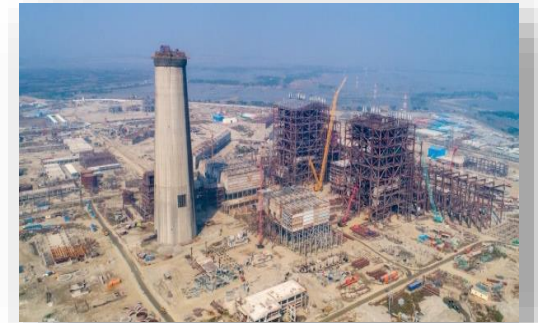
2X660 MW at Rampal, Maitree, Bangladesh-BIFPCL
