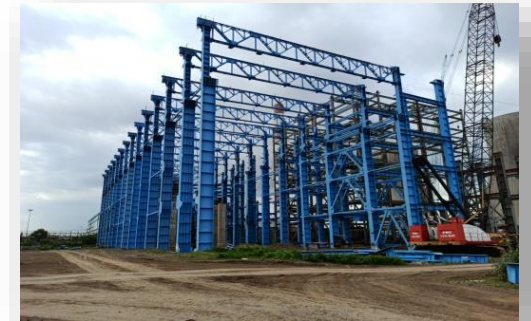
1X660 MW Bhusawal TPS at Maharastra-MAHAGENCO
