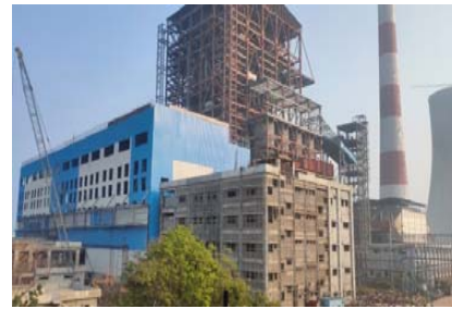
1x800 Mw TPSS, North Chennai, TNNGEDCO
