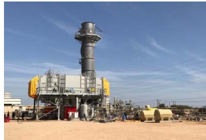
25 MW, Ray Project-RAY International LLC, Oman
