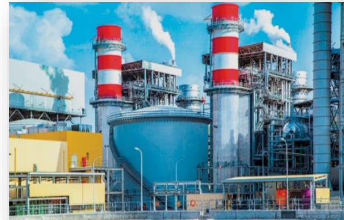
1,516 MW IBRI IPP, SEPCO – 3, Oman (Completed Project)
