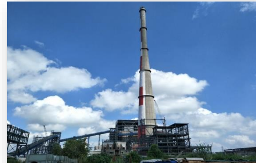
1x660 MW Harduaganj TPS, UPRVUNL
