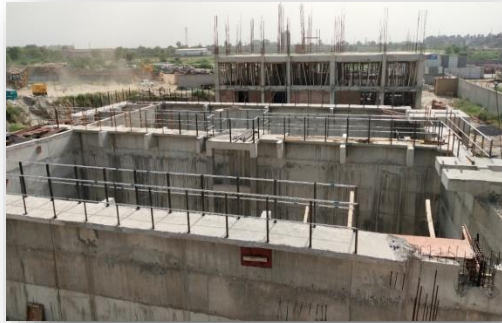
27.5 MLD STP, Networking at Palwal, MCPALWAL
