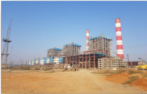
3x660 MW Nabinagar STPP, NPGCL
