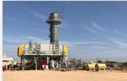
25 MW, Ray Project-RAY International LLC, Oman
