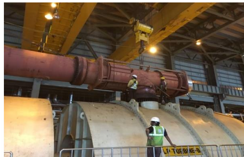
Turbine AOH, 600 MW, Udipi
