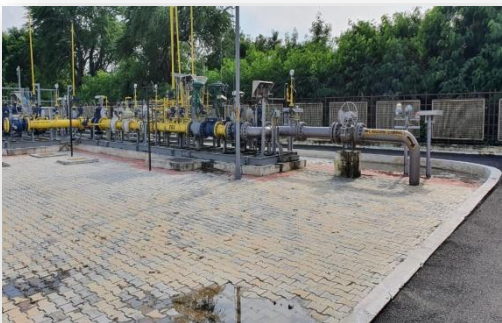
Station Piping at Ennore, IOCL
