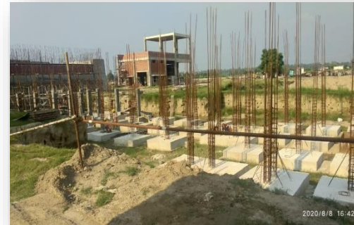
28 MLD STP at Karnal, TPL
